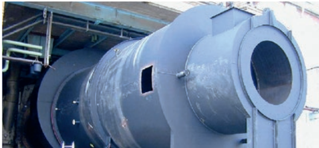
SAACKE hot gas generator during installation
