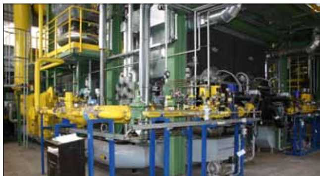
ArcelorMittal Bremen GmbH – SAACKE realized the lean gas firing system
